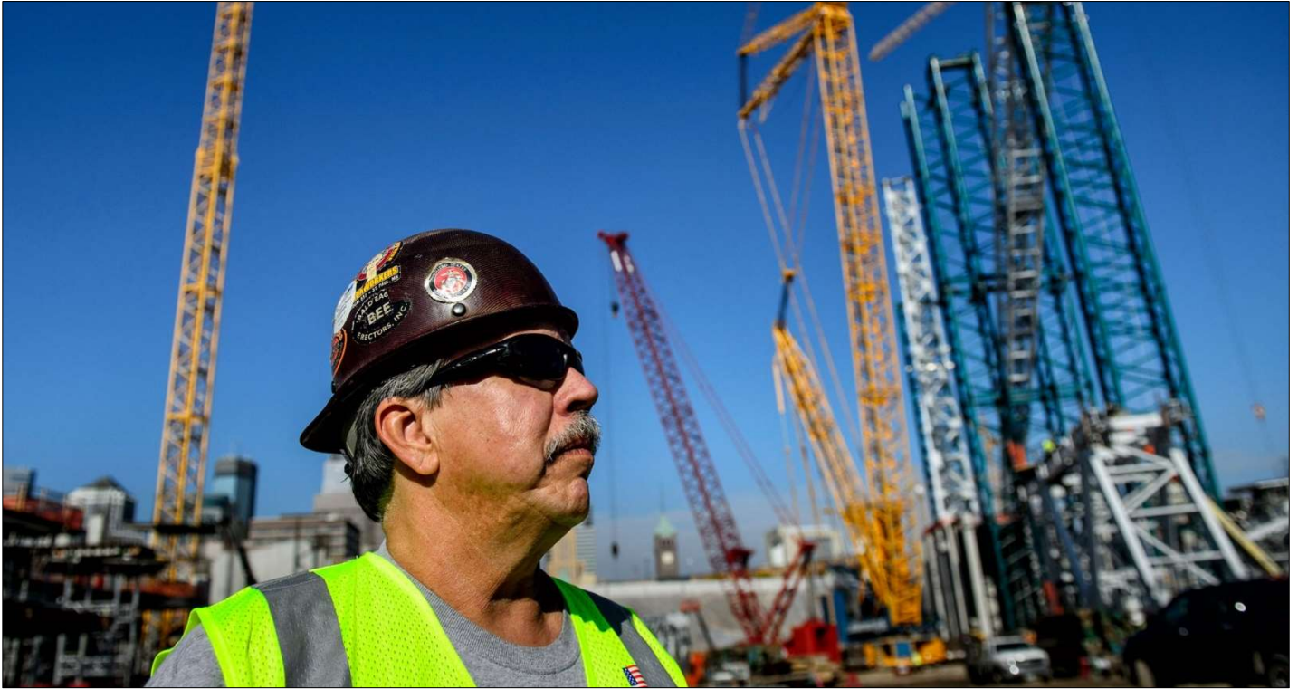
Veteran ironworker and Native entrepreneur Dave Bice (White Earth Ojibwe) successfully secured a bid for his company Bald Eagle Erectors, Inc. to help build the Minnesota Vikings National Football League stadium thanks in part to a $200,000 working capital loan from the Minneapolis Foundation. (Photo: Bald Eagle Erectors, Inc.)
